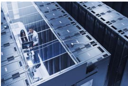
Data center power
