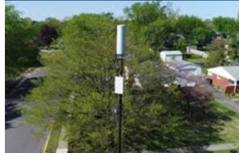
Fixed Wireless Access
