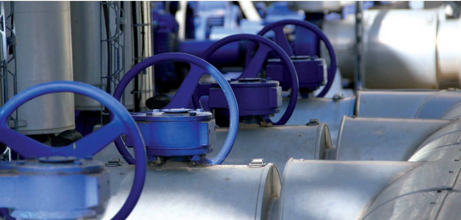
Water system, Rousset, France
